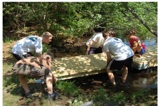
Jeremy, Brendan, Jan and Corey installed the dock at Roaring Brook Nature Center June 28 th .
